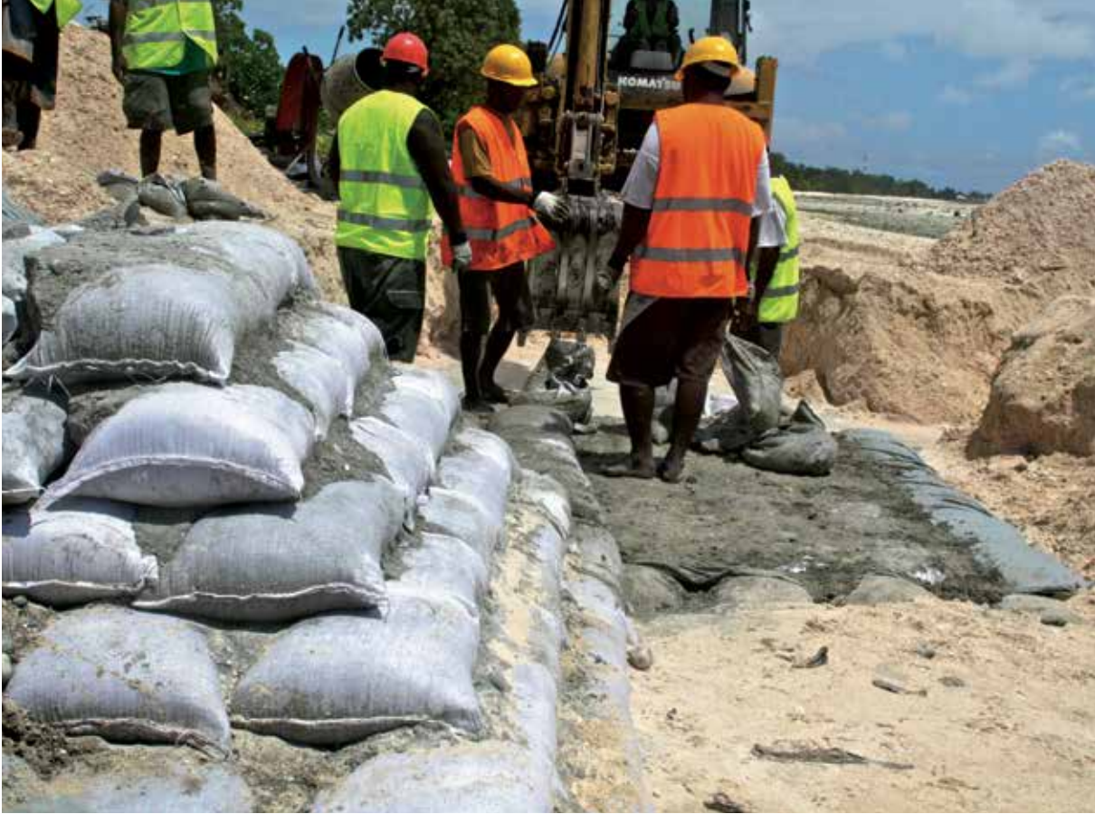
Workers constructing seawalls to prevent soil erosion in Tarawa, Kiribati (World Bank).
