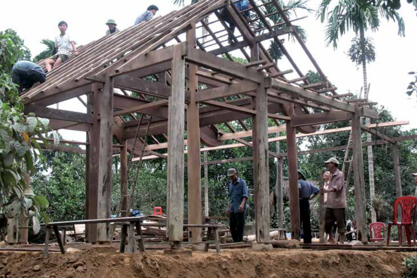
Communities in Quang Tri, Vietnam help each other to rebuild houses after severe floods (Oxfam GB).
