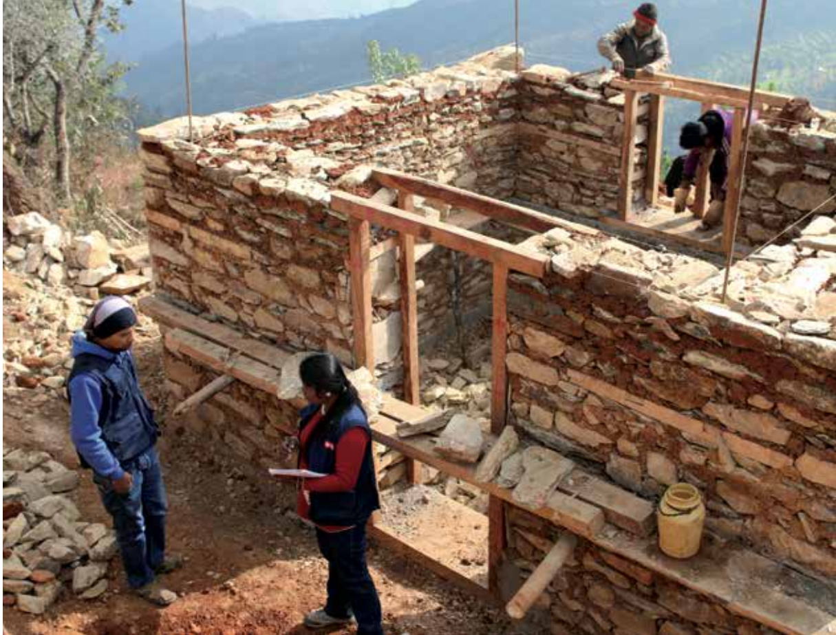
A reconstruction project in Nepal following the 2015 earthquakes that destroyed 91% of the houses in the Ramechhap district. This project seeks to build back better including through masonry trainings and improved building design (Medair).
