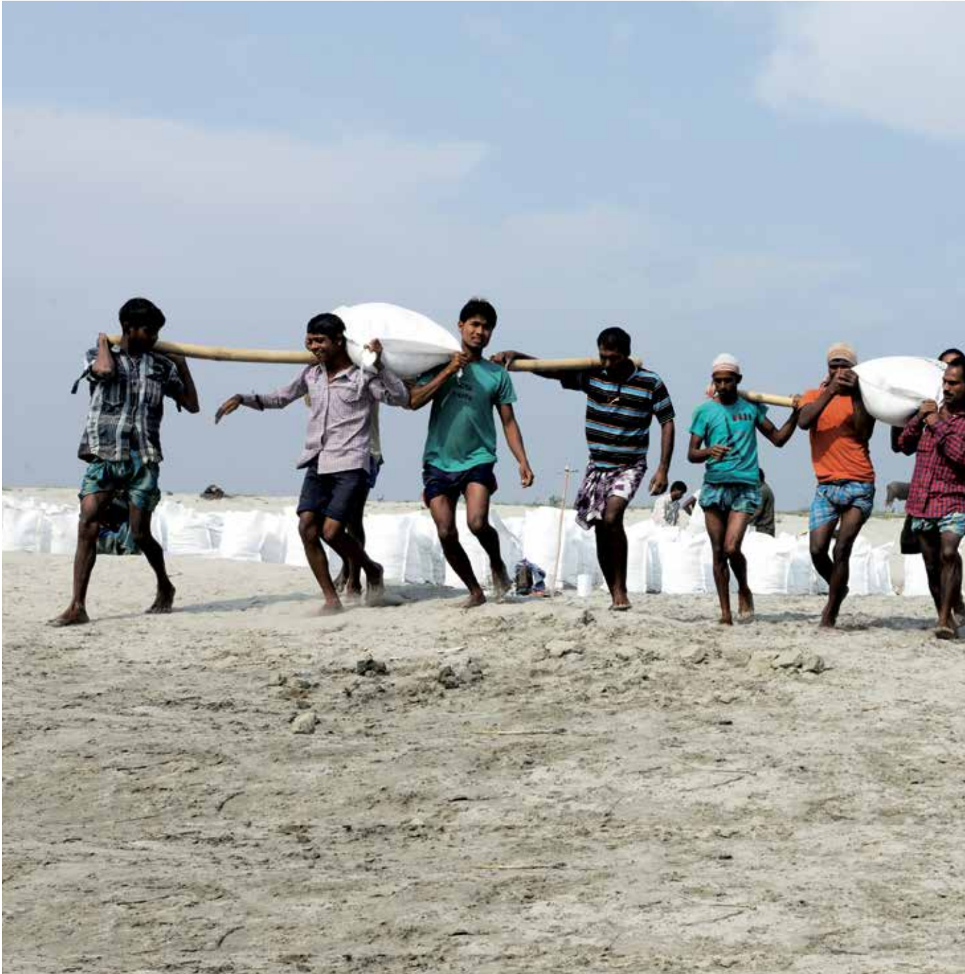
Workers carrying sand bags to be pitched on the banks of the river Brahmaputra in Gumi village, Guwahati, Assam, India. This protects the village from flooding through preventing soil erosion of the riverbank (Asian Development Bank).
